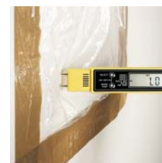
Plaster moisture contents
